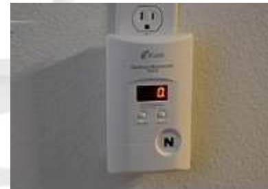
Carbon monoxide detector connected to an electrical outlet
